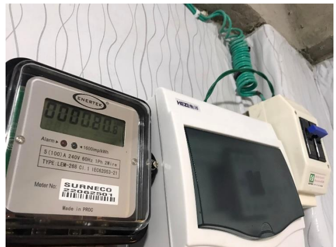
Fig. 3. Testing of Power Consumption.
